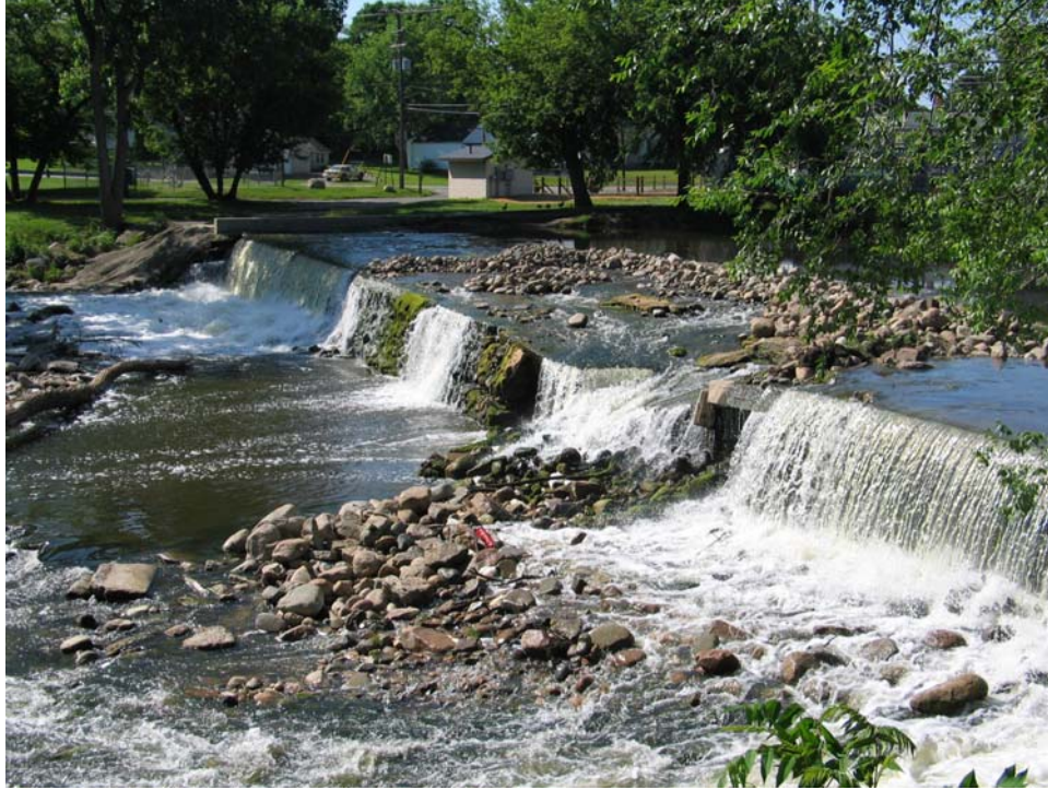
Chesaning Dam (partially failed), Chesaning, Michigan
