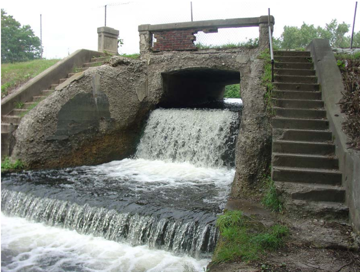
Brown's pond dam (prior to repair), Blue Lake Township, Muskegon County, Michigan
