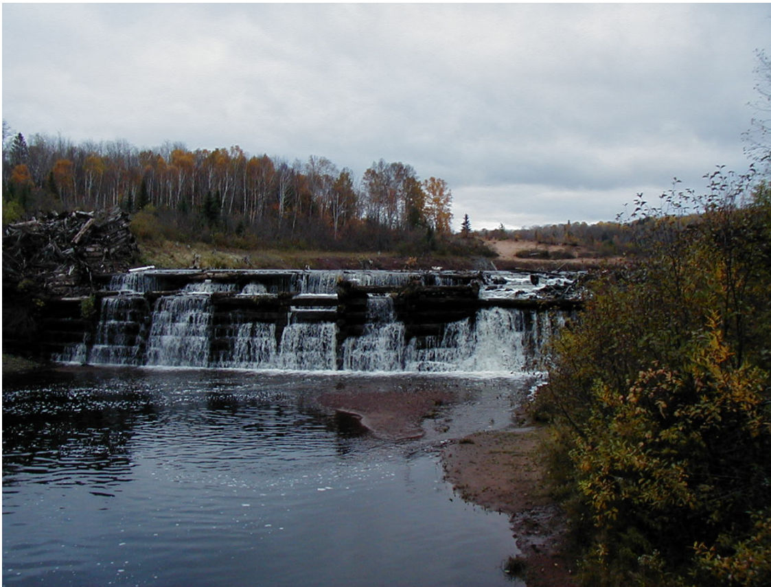
Redridge Dam viewed from downstream, after the removal of the top 10–12 feet of the dam
